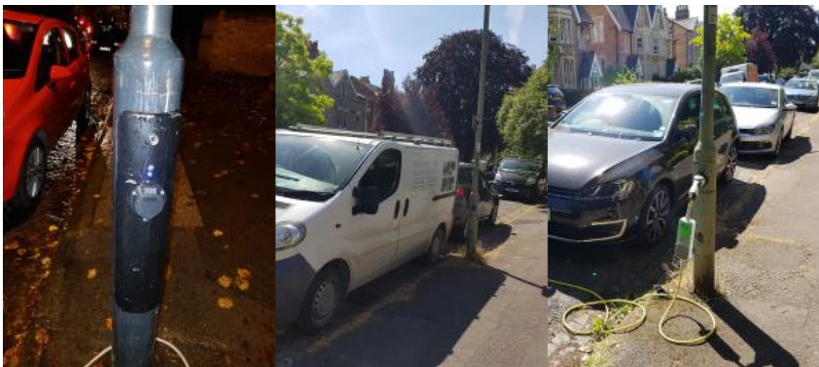
Figure 6. Three images of the Ubitricity lamppost charger which highlight how this installation by being able to be incorporated into existing infrastructure and only emitting a very small amount of light even at night, subtly integrates into the existing physical fabric of neighbourhoods. The right hand image shows how the visibility of the installation, especially for pedestrians, is enhanced when the bright yellow cable with the integrated metering system is plugged into a car. Pictures taken by: B. J. Doody.
