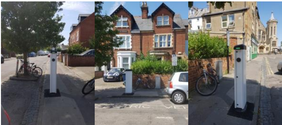
Figure 9. Three images of the e-Post charging bollard show the footprint and height of the charger itself. The central and right images capture the full footprint and two main parts of the system, the charger and the silver transformer box located in front of the brick fence. Pictures taken by: B. J. Doody.
