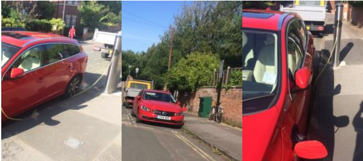
Figure 10. Three images of the Chago Pro charging station bollard show the footprint and height of the charger itself. The central image captures the full footprint and two main parts of the system, the charger and the green transformer box located in front of the brick fence. Pictures taken by: Trial participant Thomas.
