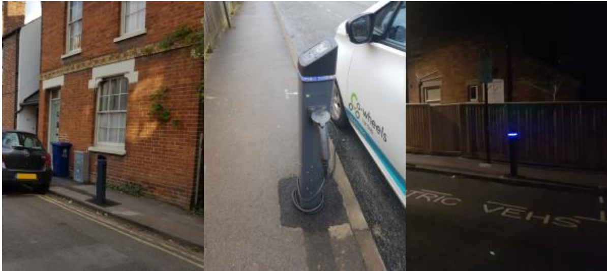
Figure 8. Three images of the Smartscape charging bollard show the footprint and height of the charger itself. The left image captures the full footprint and two main parts of the system, the charger and the silver transformer box located under the window sill. The right image illustrates how the blue glow of the charger makes it more visible at night. Pictures taken by: B. J. Doody.
