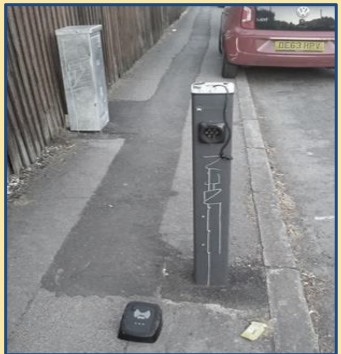
Figure 5 - A Zeta Smartscape bollard that has been vandalised and put out of service
