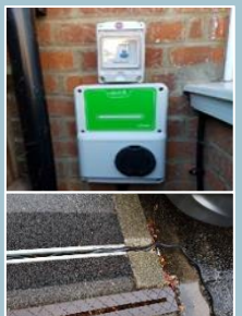
Figure 3: On-street charging technologies included in the Go Ultra Low Oxford trial.
