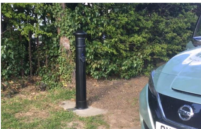
Figure 17 – Example of Ubitricity bollard installed close to, and drawing power from lampposts in some locations.
