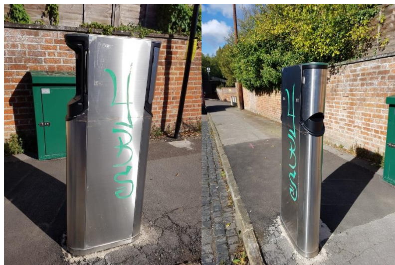
Figure 8. A side and front view of a Chago Station charging bollard of the damaged caused by a vehicle driving or reversing into the front of the charger. The image on the left illustrates that this accident has removed the door on the left side of the charger. According to Thomas this has rendered this port unusable. The right side port continues to function. Pictures taken by: B. J. Doody.
