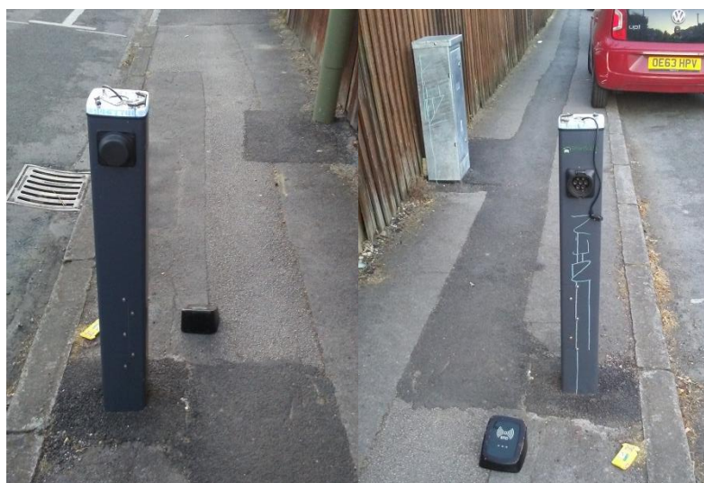
Figure 9. Two separate views of the side of a Zeta Smartscape Charging Bollard which has had the top of the unit removed by what appears to be an intentional act of vandalism. Pictures taken by: Oxford City Council Staff.
